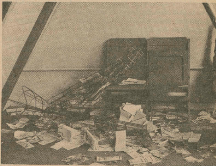
The front room of the office contained materials scattered from the explosion. At left, the partition with a door leading to the backroom leans forward supported by a brace.
