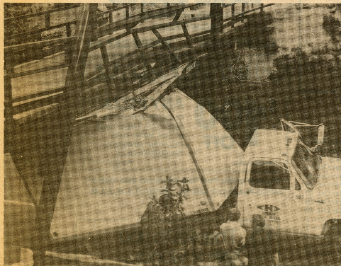
The impact wrenched the bridge, cracked the foundation and bent the undercarriage of the truck.
