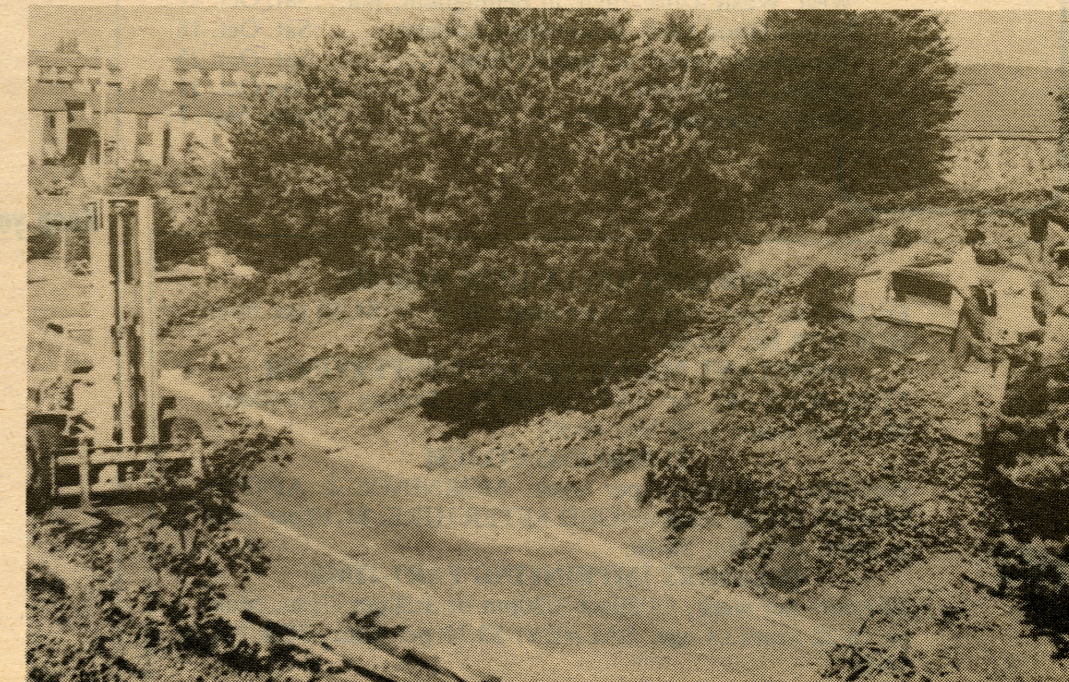
Part of the construction job was tearing down the old structure. photo by C.P. Stancich
